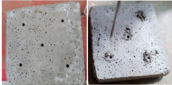
Figure 8 Screwing effect on ceiling panels
