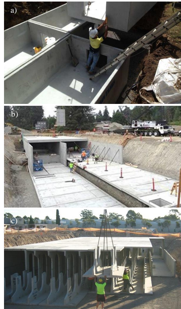
Figure 3 Types of stormwater storage structures, a) Tanks [8], b) Panels [9], c) Modular Units [10]
