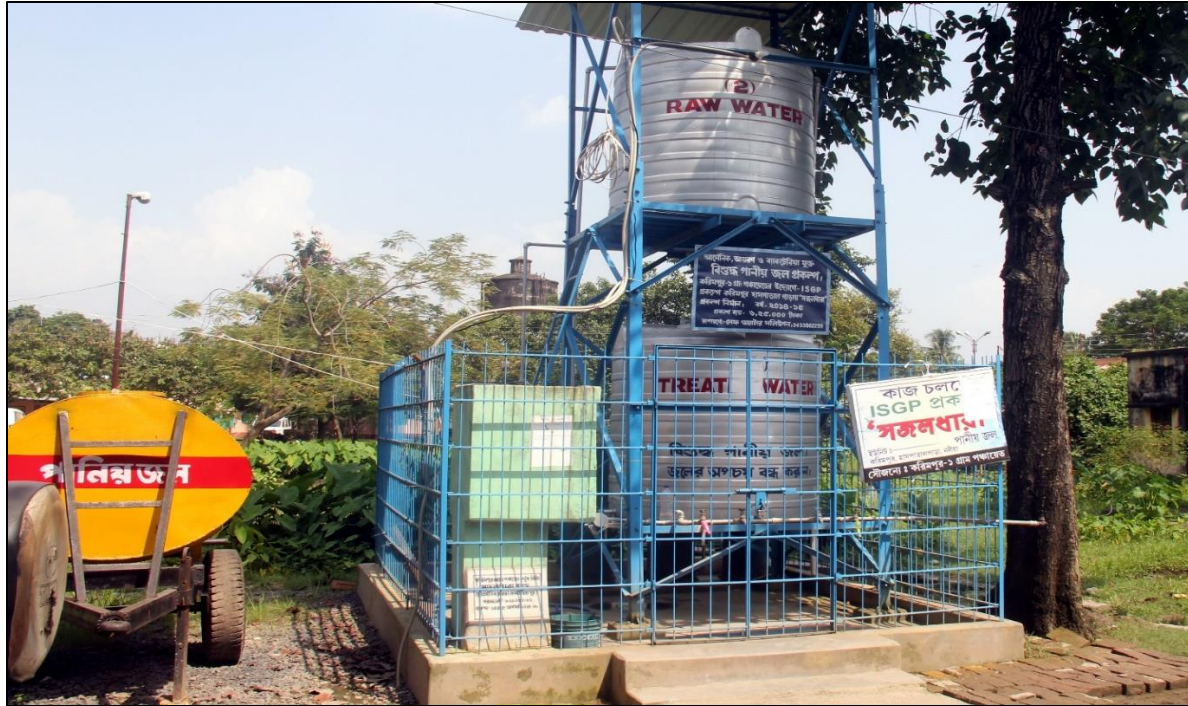
Figure 9 Water tanker to supply drinking water to distant households
