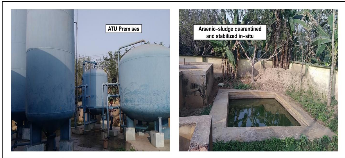
Figure 11(a) Wastewater generated by an ARP located in School Para habitation of the Mrigipota village under Chapra block in district Nadia, commissioned scheme under Bahirgachhi Water Supply Scheme (Zone-2)
