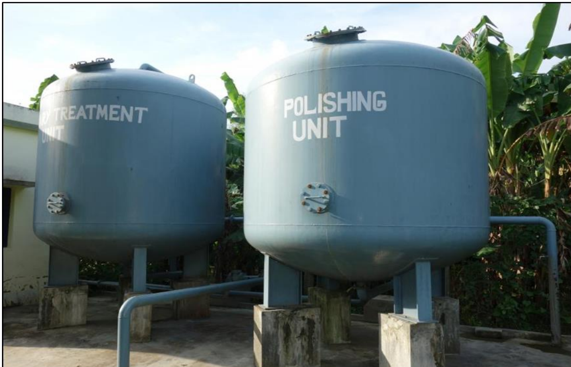
Figure 5 A typical ATU located in doctor para habitation of the Khanjepur village under Tehatta-I block in district nadia, commissioned scheme under Khanjepur water supply scheme
