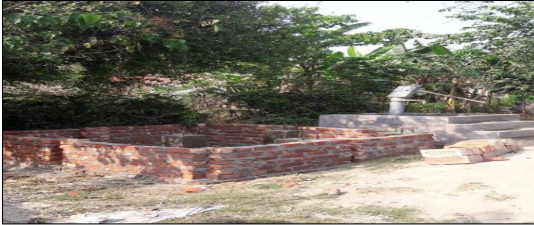
Figure 14 Clay-bricks being used for construction of an ARU in rural West Bengal (location Gosaichar Purbapara habitation of the Gosaichar village under Ranaghat-I block in district Nadia, GP Nawpara Masund)
