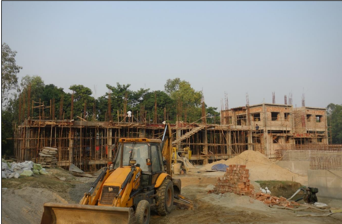
Figure 13 A construction site in Gangarampur Municipality in district Dakshin Dinajpur, utilizing value-added construction materials incorporating waste products such as agricultural residues and municipal wastewaters
