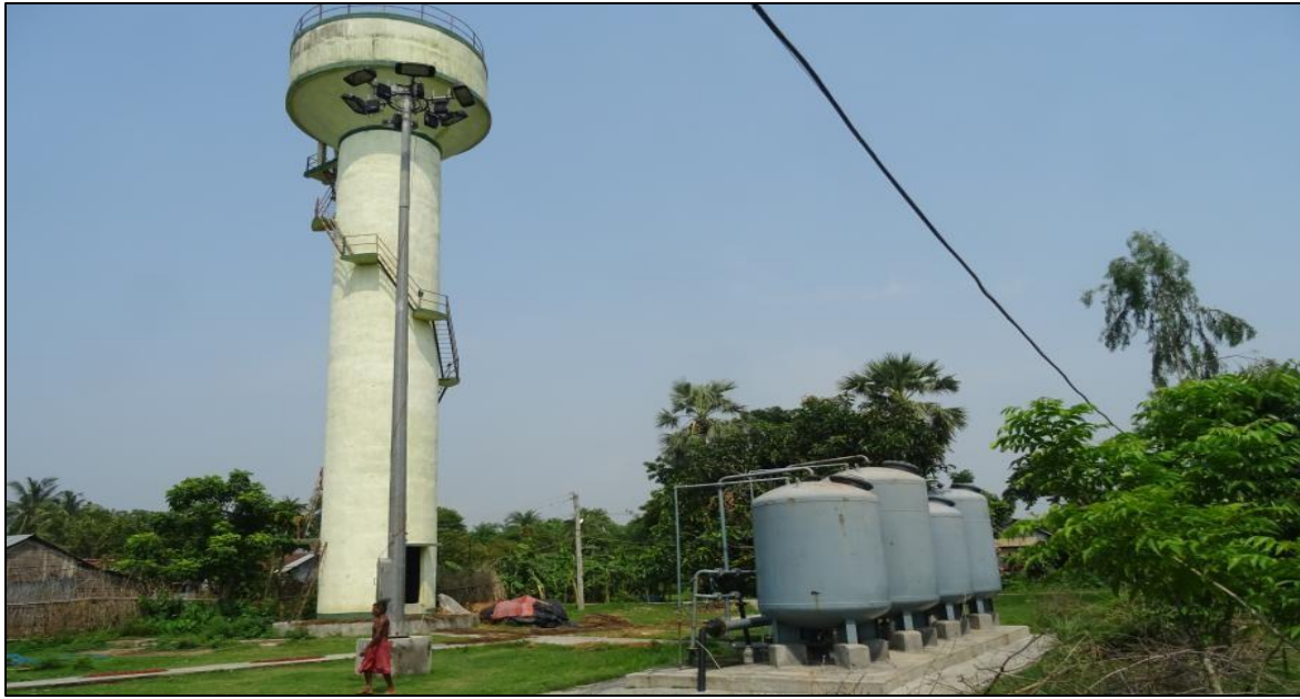
Figure 7 A typical ARP located in Char Panpara habitation of Panpara village under Shantipur block in district Nadia, commissioned scheme under Gayespur Water Supply Scheme (Zone-2)
